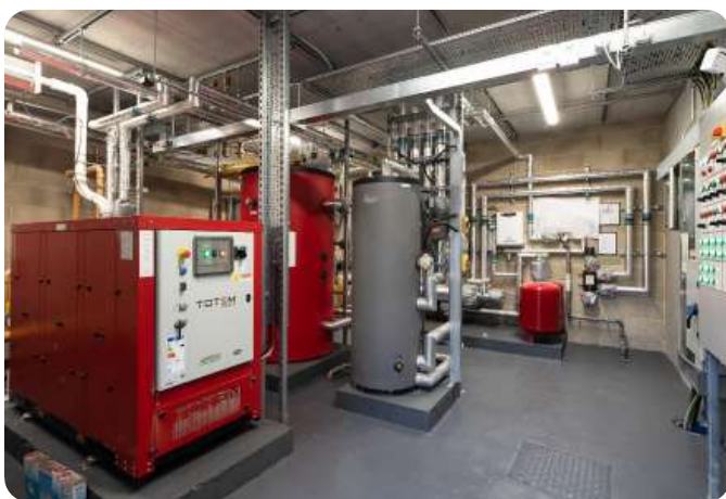
Fig.227. Efficient plant room design Levitt Bernstein
