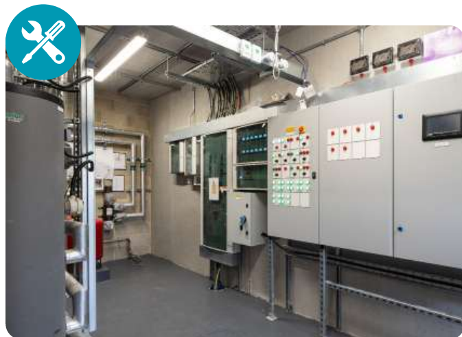
Fig.112. Plant room with adequate space for replacement Levitt Bernstein
